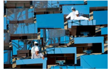
Figure 25.12. Two engineers assembling an eSolar concentrating power station using heliostats (mirrors that rotate and tip to follow the sun). esolar.com make medium-scale power stations: a 33 MW (peak) power unit on a 64 hectare site. That's 51 \text{ W/m}^2 peak, so I'd guess that in a typical desert location they would deliver about one quarter of that: 13 \text{ W/m}^2 .
