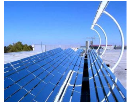
Figure 6.19. A combined-heat-and-power photovoltaic unit from Heliodynamics. A reflector area of 32 \text{ m}^2 (a bit larger than the side of a double-decker bus) delivers up to 10 kW of heat and 1.5 kW of electrical power. In a sun-belt country, one of these one-ton devices could deliver about 60 kWh/d of heat and 9 kWh/d of electricity. These powers correspond to average fluxes of 80 \text{ W/m}^2 of heat and 12 \text{ W/m}^2 of electricity (that's per square metre of device surface); these fluxes are similar to the fluxes delivered by standard solar heating panels and solar photovoltaic panels, but Heliodynamics's concentrating design delivers power at a lower cost, because most of the material is simple flat glass. For comparison, the total power consumption of the average European person is 125 kWh/d.
